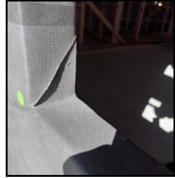
STEP 3: Fold main underlay flaps over "insert" and fix in place. Tape window as per Step 4-9 on page 10.
