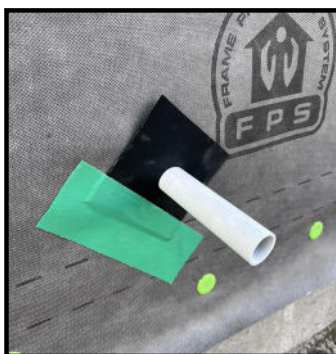
STEP 2: Remove one side of the split backing paper from the ES60 Tape, place the exposed adhesive side onto the FPS® Seal, ensuring equal lengths of ES60 Tape extend beyond each end of the FPS® Seal.
