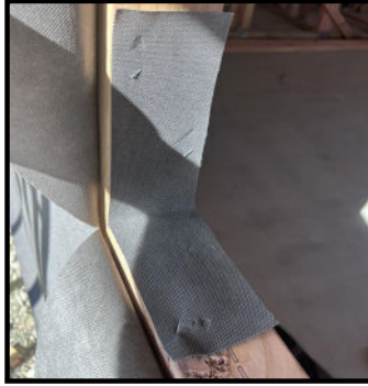
STEP 2: Insert section into corner of frame with equal length up and across frame. Fix in place with staples.
