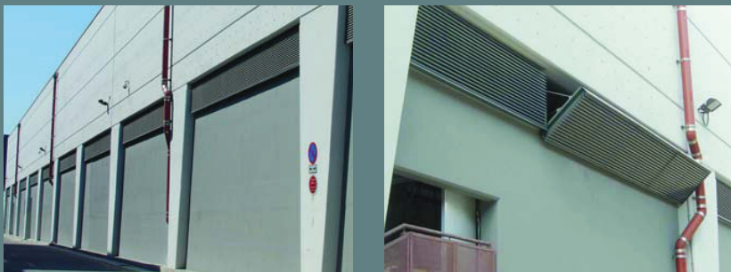
Mass Transit Railway Corporation (MTRC), Hong Kong. Side vents fitted externally with Colt Universal Louvre in line with surrounding Colt Louvre panels.
