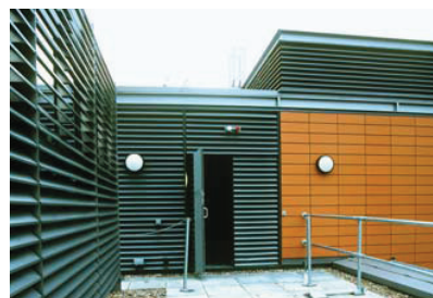
Evelina's Childrens' Hospital, London. Plant room louvres and doors.
