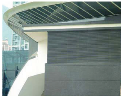
Indoor Recreation Centre, Ma On Shan, Hong Kong. Universal Louvre for plant room ventilation and for controllable air inlet for the smoke extraction system.
